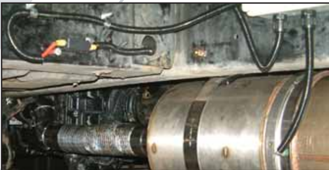
Battery supply wiring including 30 Amp fuse Fig 14
